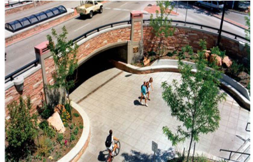
Figure 4.g: Use of appropriately scaled materials enhance the pedestrian environment of this underpass.
