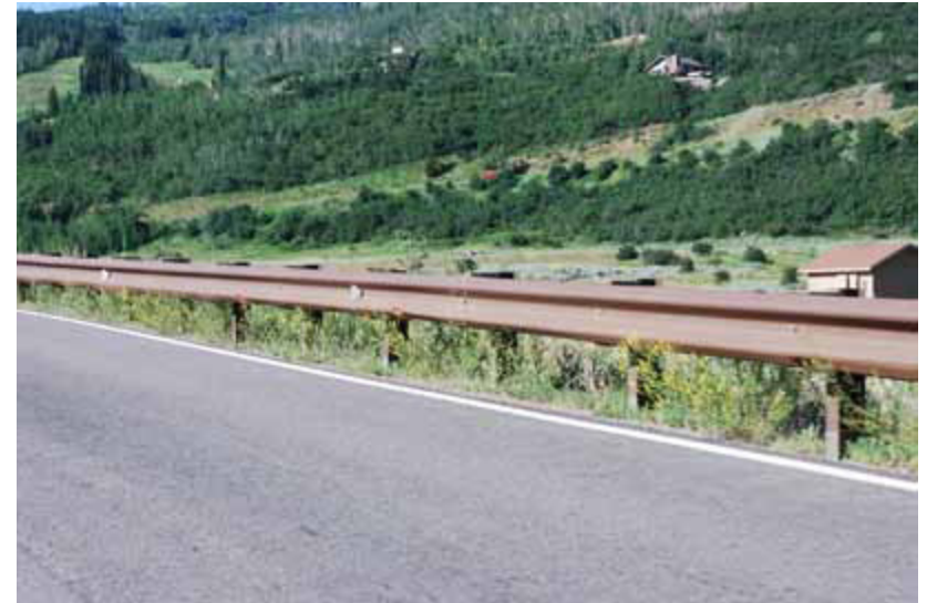
Figure 3.zg: This simple barrier design with rusted metal rails and wood posts blends well in its setting.
