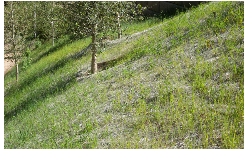
Figure 2.w: A variety of techniques are used in this urban setting. They include chain link fencing for site protection, straw erosion control matting and black silt fencing to trap sediments.
