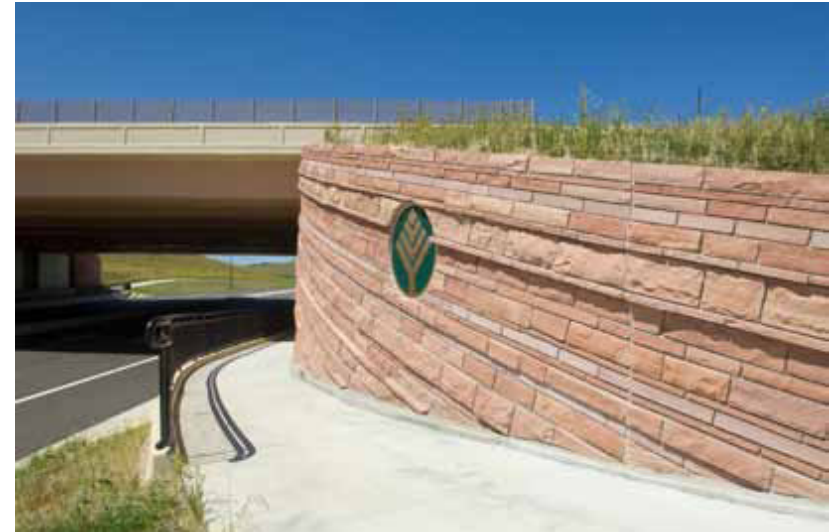
Figure 3.y: The retaining walls are curved to become well integrated with the adjoining slope.
