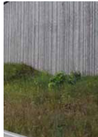
3.w: The fluted formwork of this concrete wall creates a visually simple texture that renders a shadow pattern on the surfaces.
