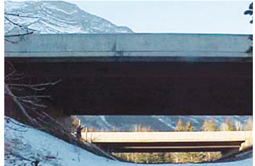
Figure 2.f: This raised roadway crossing over a natural drainage provides a wildlife movement corridor.
