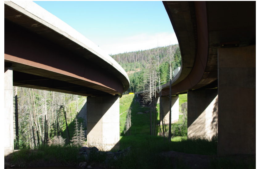
Figure 2.h: This bridge is raised high enough for naturally occurring vegetation to be preserved.
